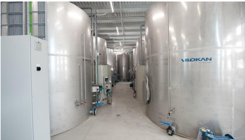
Step 4 – cont'd Quality-control tanks.
